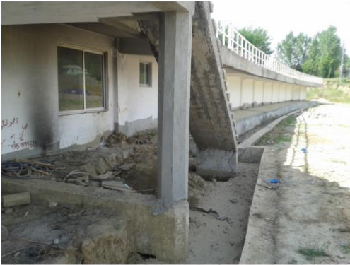
Footpath and drain incomplete
