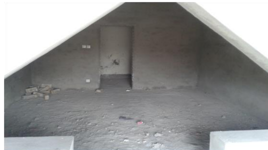
Inappropriate size and location of door in office
