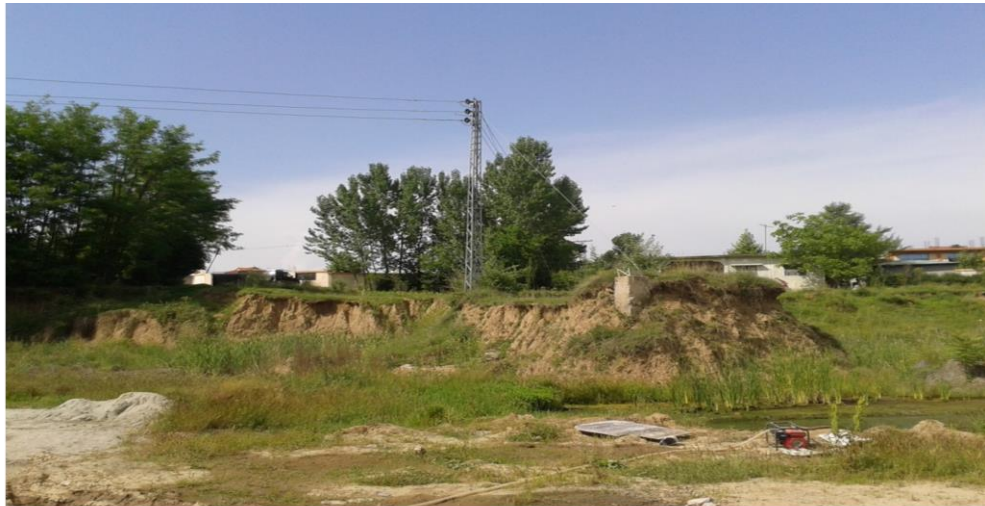
Electric Pole required to be shifted to facilitate the construction of Parking and approach road
